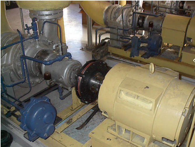
MGE-11, 50HP, 3600RPM HVAC, Hospital, Salt Lake City, UT
