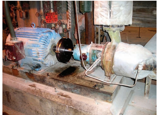
MGE-11, 100HP, 3600RPM, Pulp & Paper Plant, Clean Condensate Pump, St. Helens, OR
